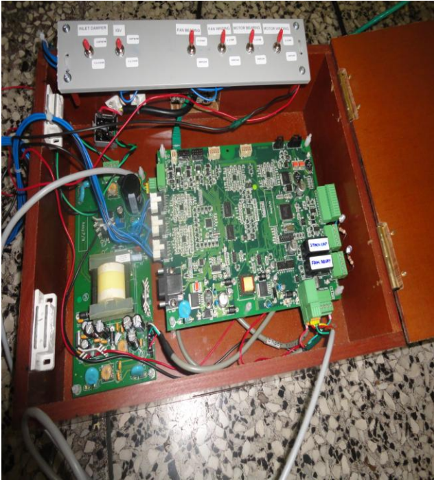
Fig-2 Hardware Components
