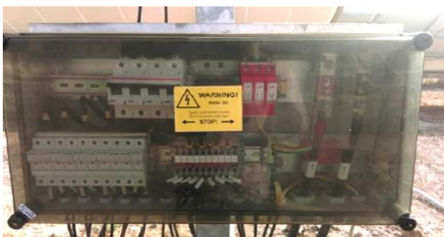
Fig.1.3 Snapshot of DC Distribution Box
