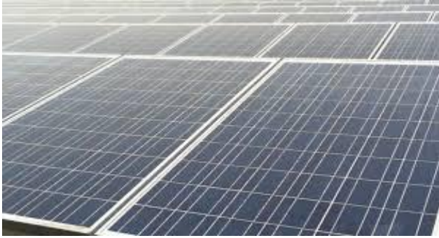
Fig.1.2 Snapshot of Installed Solar PV Plant Table-1Description of Solar Panel
