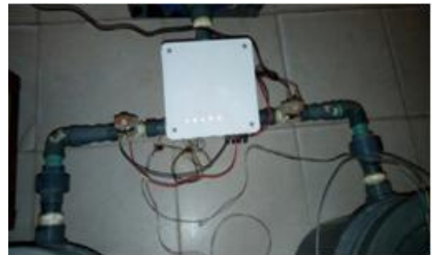
Figure 12: Casing with the LED Indicators Water Level Monitoring System
