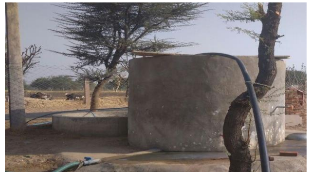
Fig. 13. Solar PV water pumping system installed at Jaipur (Rajasthan)
